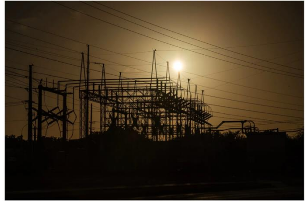
A power station in Corpus Christi, Texas. Photographer: Eddie Seal/Bloomberg
